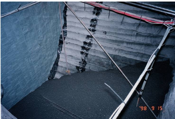
Figure 3. Pouring a keyed concrete bulkhead for the Tunnel Sealing Experiment in Canada (Read 2008).
